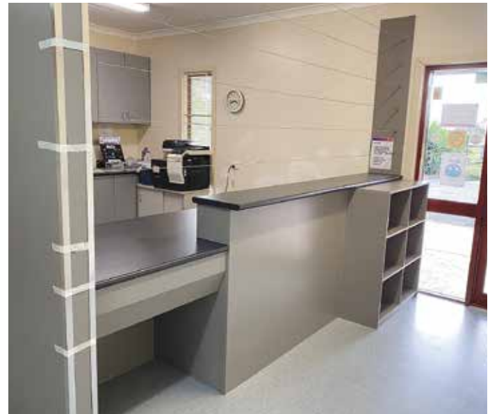
Delivery Campaspe Animal Shelter Facility Improvements Upgrades are underway at the Campaspe Animal Shelter which include sound proofing, a new reception area, new shade sails in the dog outdoor play area and a new synthetic grass play/meeting place.
