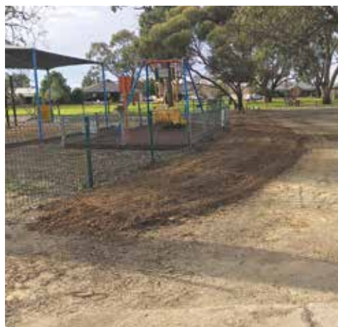
Completed Shire Parks and Playgrounds Irrigation renewal Irrigation works at John Pilley Reserve at the entrance to the Kyabram Fauna Park were completed in May.
