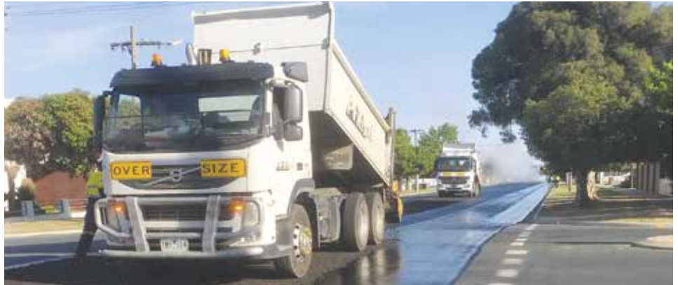
Resealing works on Hare Street, Echuca - part of this year's Sealed Road Resurfacing Program.
