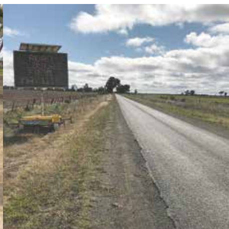
Delivery Corop Wanalta Road Reconstruction, Burrumboot Road works on a section of Corop Wanalta Road have started and are anticipated to be finished by late June.
