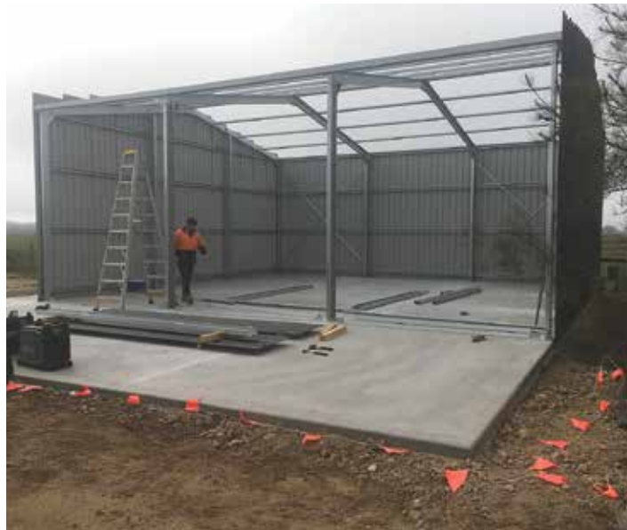
Delivery Transfer Stations, e-waste Compliance Facility Installation E-waste facilities at Rochester, Kyabram, Toolleen, Colbinabbin and Rushworth are under construction. With Gunbower and Lockington facilities already completed.
