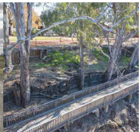
Procurement/Delivery Echuca Murray Esplanade Retaining Wall The contract has been awarded and construction of a 65 metre section of new retaining wall started in May, north of the Echuca Wharf.
