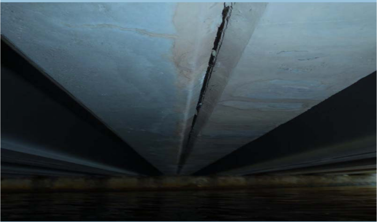
Staining btw 'U' slab units indicating shear key failure
