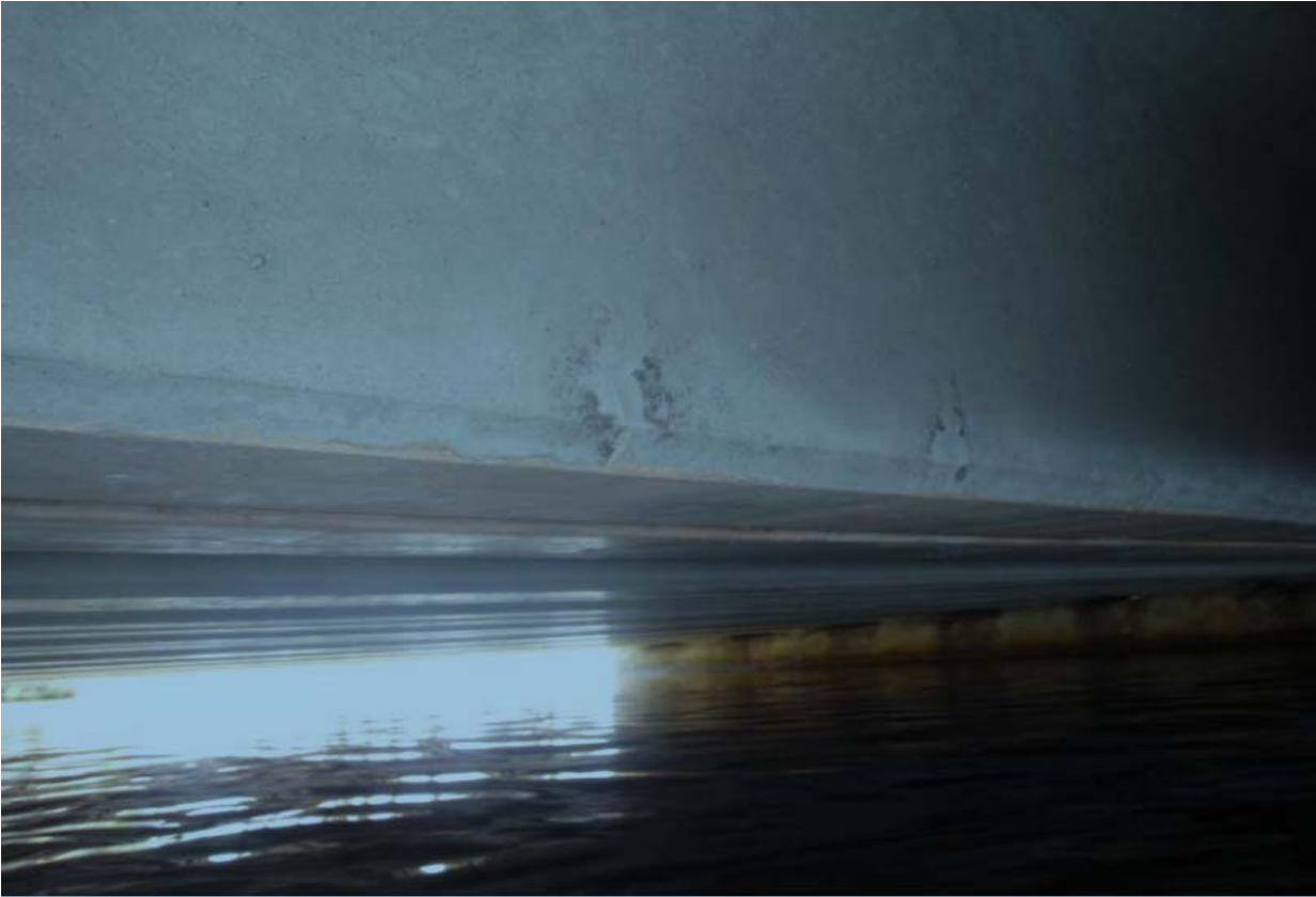
Fine flexural cracking
