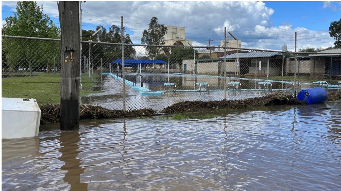
Figure 4: Rochester Pool Flooding Impact (Source: Shepparton News, 2022)
