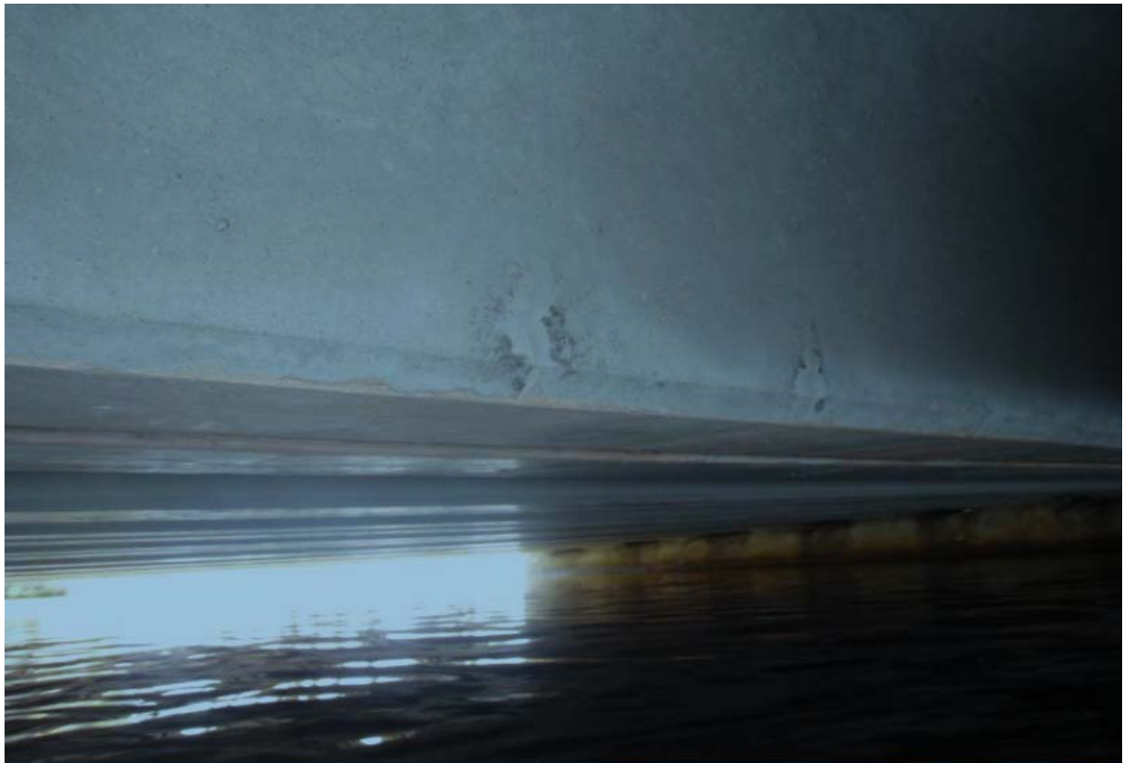
Fine flexural cracking
